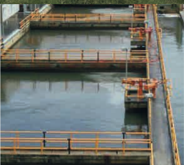
Designs and technical advising for the construction of the Francisco Wiesner Treatment Plant Colombia
